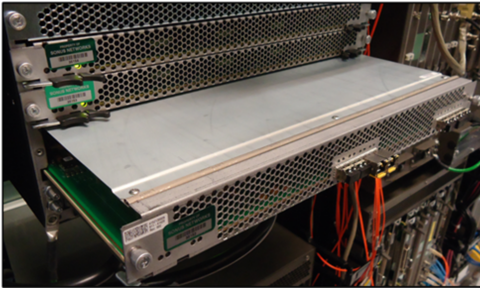
Figure 2: SBC 7000 Core Server Card pulled out
